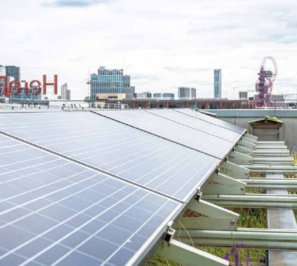
Solar panels on the Press Centre roof feed back into the building's power supply, generating enough electricity to power 27 homes.
